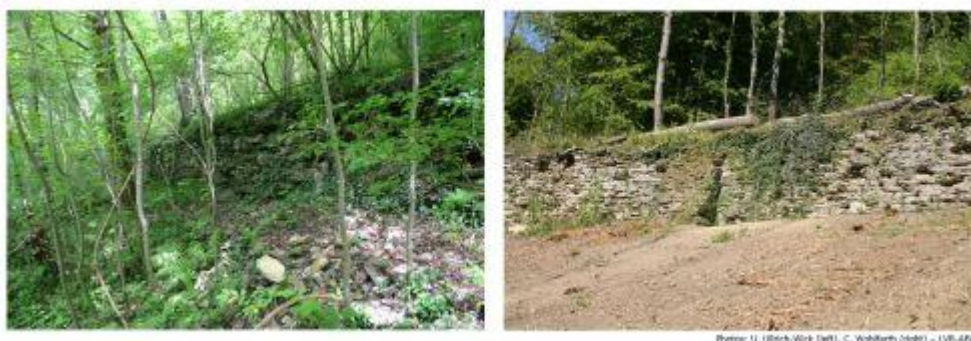
Figure 14: 'Hager Weinberg' before and after cleaning from damaging vegetation (Image credit: U. Ulrich-Wick, C. Wohlfarth – LVR-ABR)
