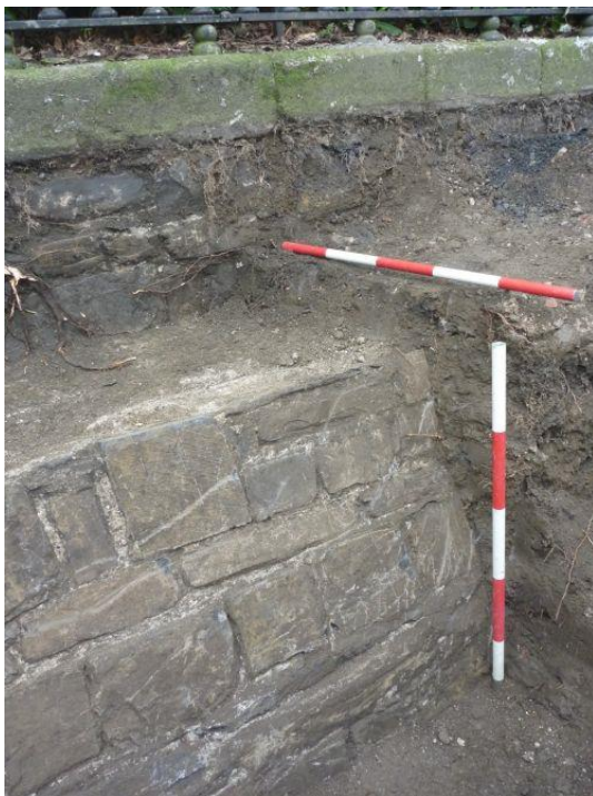
Figure 14: View of the retaining revetment wall of St Stephen's Green Park's perimeter ditch (or ha-ha). Note this wall now functions as the foundation for the Park's perimeter fence (Rubicon Heritage Ltd)
