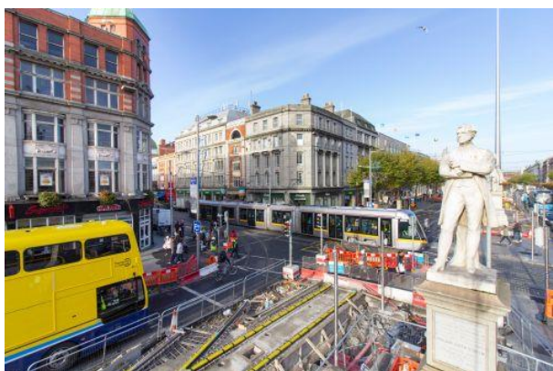
Figure 7: O'Brien National Monument on O'Connell Street, showing LCC construction works and an inbound Luas Red Line tram (Transport Infrastructure Ireland)
