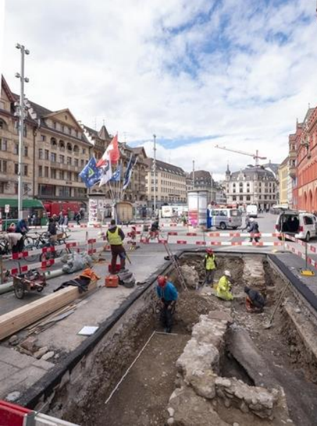
Figure 1: In 2022, the remains of a row of houses, which had fallen victim to a devastating fire in the 14th century, came to light on Marktplatz, Basel, Switzerland.
