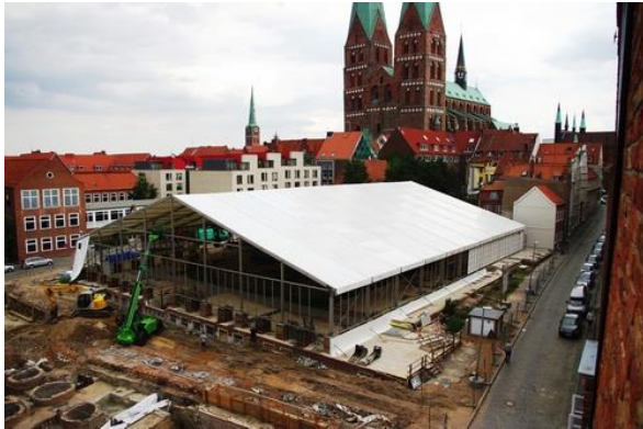
Figure 6: A large excavation tent was erected over the demolished school buildings, allowing the archaeological work to proceed regardless of the weather, temperature and season. In the lower left part of the photo, the brick cesspits in a backyard, which were uncovered directly beneath the parking lot, are clearly visible (© Hansestadt Lübeck, Abteilung Archäologie).
