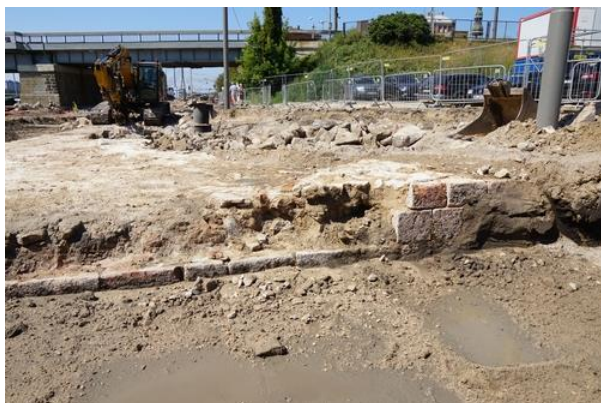
Figure 12: A fragment of the Šēra Bastion discovered during reconstruction of a street. (Photo: National Heritage Board)
