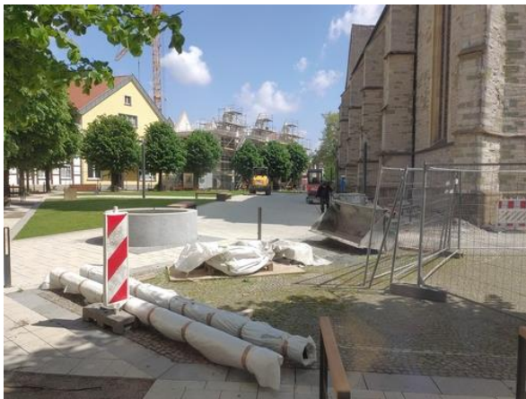
Figure 5: The almost completed St Stephanus Church Square, with upgraded substructure and extended paving. Copyright: LWL-AfW, A. Wunschel.
